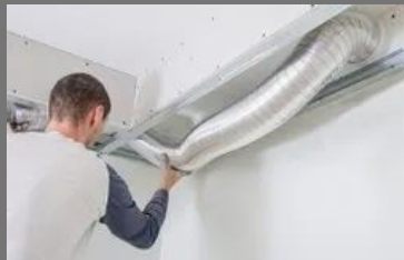
Ducting Insulation Services
